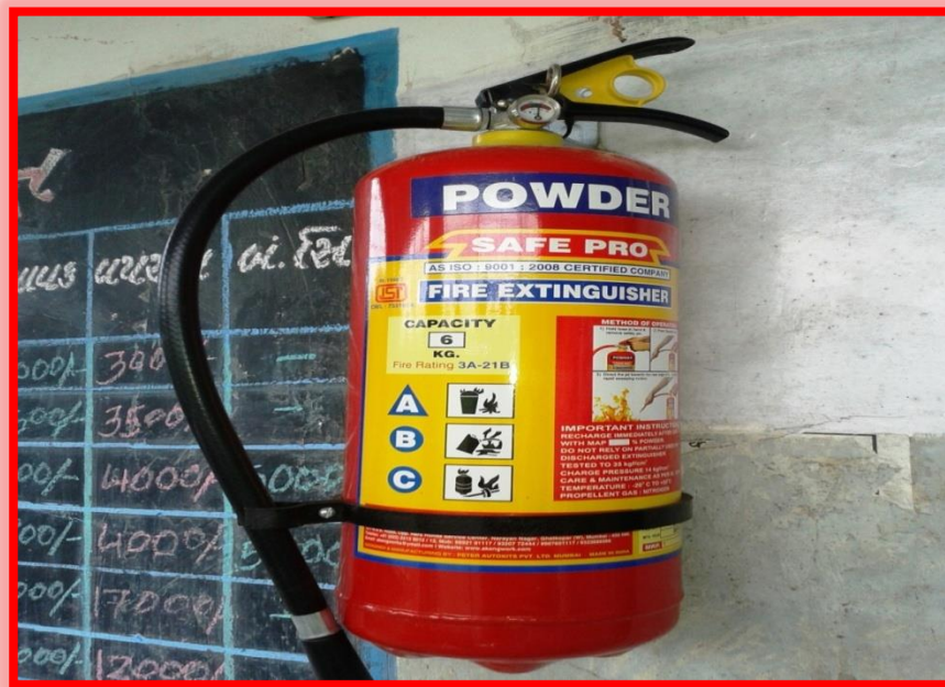
MDM: Fire Extinguisher in working condition.
